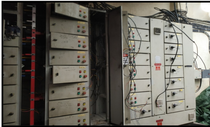
Figure 7. Electrical Panel Board.
